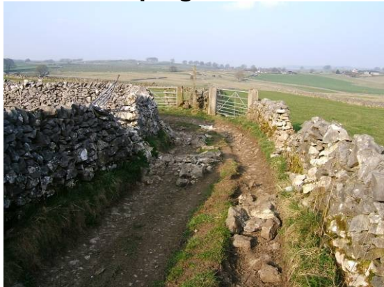
Damaged walls at Monksdale Lane, Tideswell – April 2011 (these have now been repaired)
