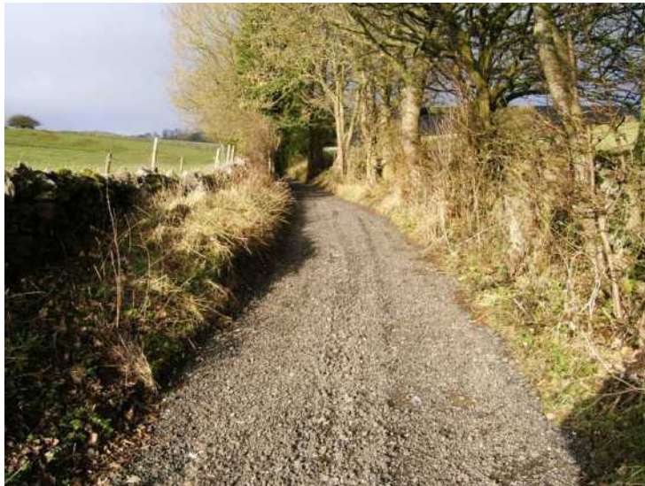
Photo: Leys Lane after the recent DCC repairs which have improved the surface and have tried to improve the drainage. December 2012
