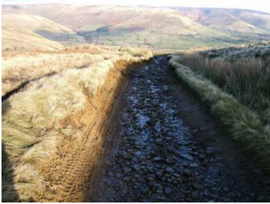
December 2012. Tracks on the side of the bank. (this area not repaired by DCC)
