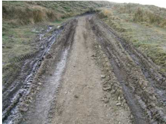
January 2013. The same area with both deeper ruts on the track and more ruts on the verges.
