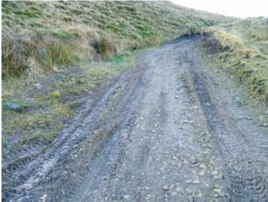
December 2012. Ruts starting to form on the left hand verge
