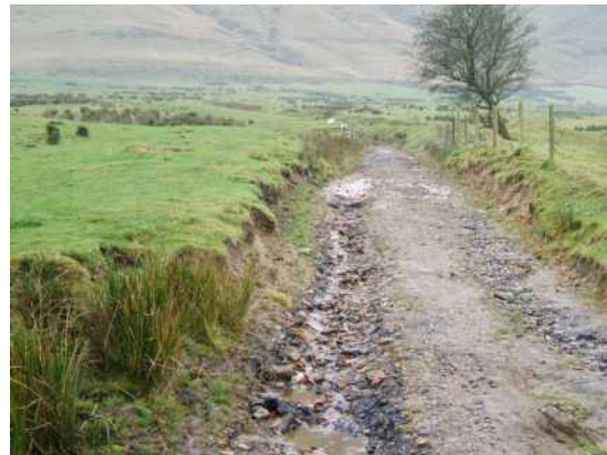
November 2012 – Damage due to run off water with no off-roading
