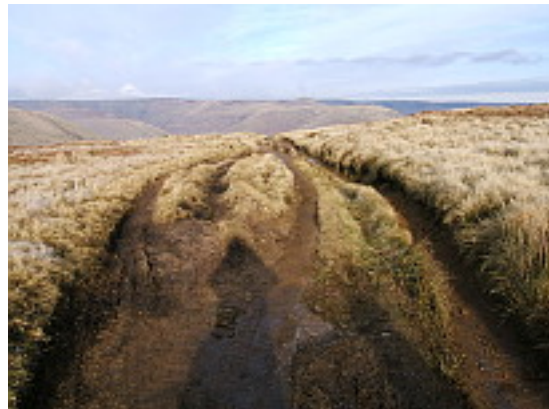
Multiple ruts on the flat plateau area that is not part of the DCC repairs. January 2013
