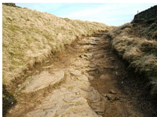
Chapel Gate eroded to bedrock on the descent to the Chapel Road. This part is not subject to DCC repairs. January 2013
