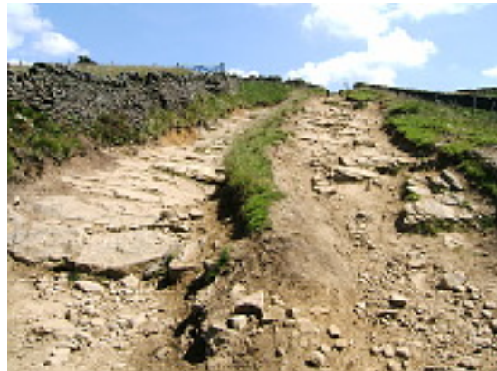
The parallel track (on the right) is now nearly as badly eroded as the main track (on the left.) DCC had a temporary TRO on the route to carry out repairs earlier this year. We could see no signs of any repairs when visiting this month. Photo: July 2013
