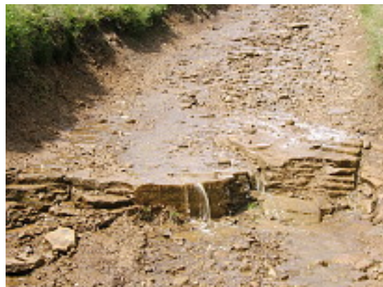
Steps are beginning to form also on the ascent to the north of Roych Clough. Water erosion is not helping. We watched a 4x4 sending clouds of dust into the air while trying repeatedly to get over a similar small step. Photo: June 2012
