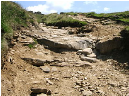
The worst of the "steps" when descending Roych Clough. Many vehicles are unable to manage this step and illegally leave the path creating a parallel track (seen on the right of the photo). Other vehicle users bring ramps to cope with the step. Photo: July 2013
