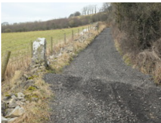
Wall damage which local people believe is due to off-roading. Photo: February 2013
