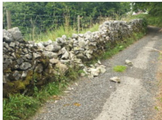
Wall damage in the narrowest part. Photo: August 2013
