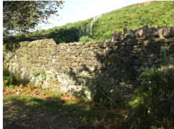
Loss of coping stones from the wall. We were told that off roaders have removed them to fill in ruts.
