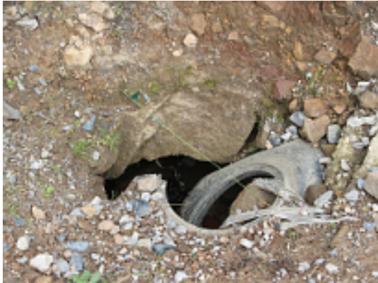
Close up view of collapsed culvert which is on the track. September 2013
