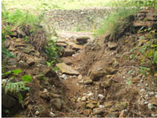
Where the run off water has washed away the wall. September 2013
