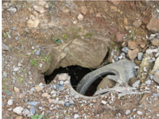
Close up view of collapsed culvert which is on the track. September 2013
