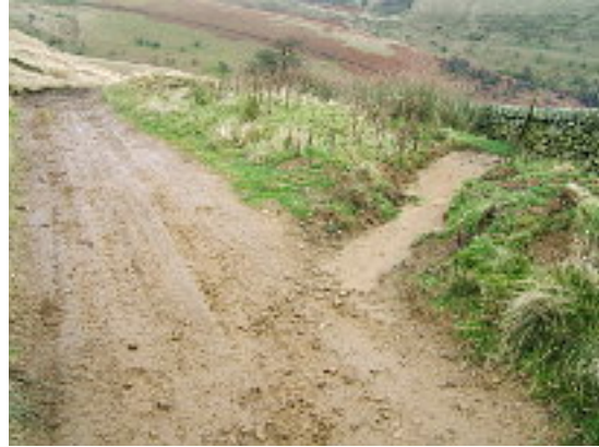
New drainage already silting up. December 2013
