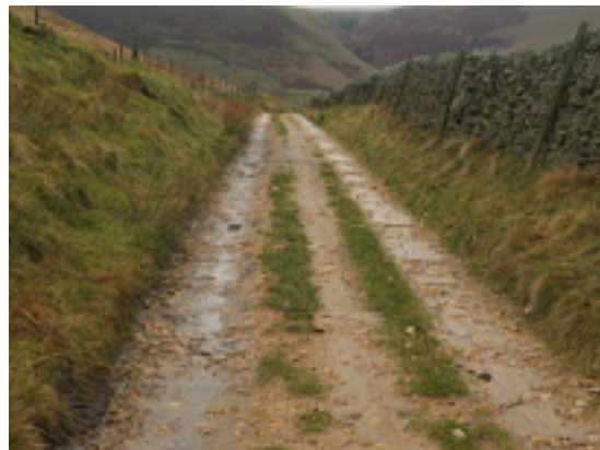
Grass is continuing to regenerate on those stretches where DCC has left the 2011 repair surface intact. Photo: January 2014
