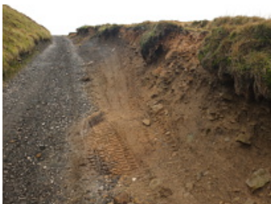
Tyre tracks on the side of the earthen bank. This is unnecessary. Photo: January 2014
