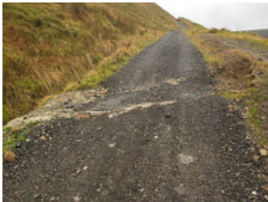
However, planings are collecting in the culverts which will need cleaning regularly if they are to remain effective. Photo: January 2014
