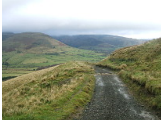
Many felt that planings were not a sympathetic material to use for the 2nd DCC repairs. However, they are wearing well where DCC has improved the drainage. Photo: January 2014
