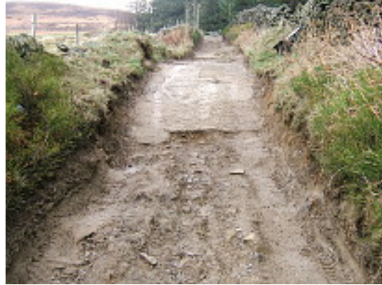
Bamford Clough. Some of the concrete which is hazardous to all users when wet that DCC plan to remove. Photo: January 2012
