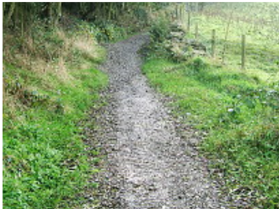
Chapel en le Frith BOAT 182 - The central section which we believe has been repaired. Photo: November 2013
