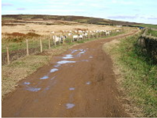
Brough Lane. Repairs carried out some years ago near where the route joins Abney Restricted Byway 5 and Duper Lane. This area used to be a mud bath. Photo: November 2012
