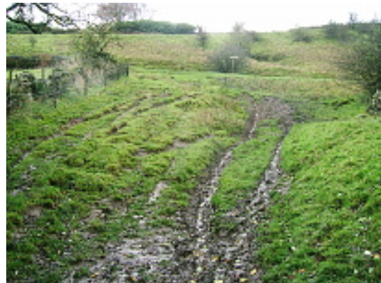
Chapel en le Frith BOAT 182. This will need repair if we have a wet winter and if it is extensively used for off roading. Photo: November 2013
