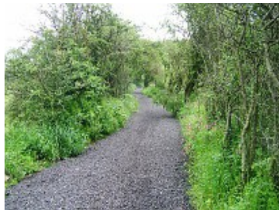
Part of the lower section (previously always muddy) when the repairs were completed in June 2012
