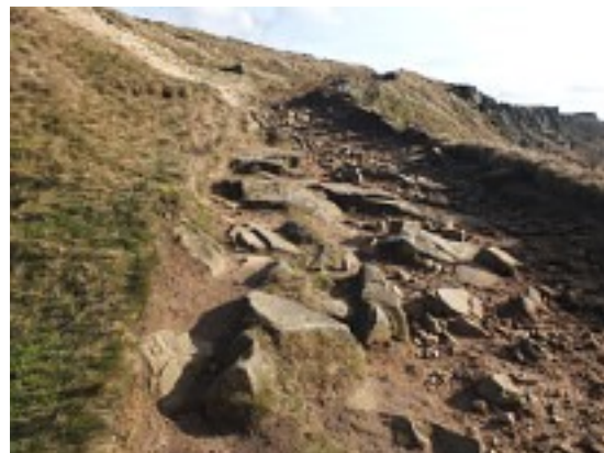
An unrepared section of Long Causeway. Photo: February 2014
