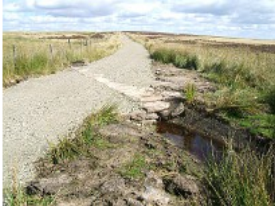
New drainage underneath the surface where a pipe leads water to a new "wetland area"
