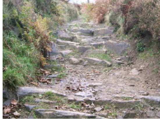
Note how the route is sunken and narrow which can make it difficult for users to get out of the way of vehicles. October 2014
