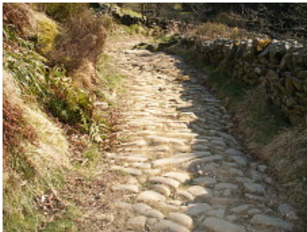
Setts needing specialist knowledge to repair. March 2016
