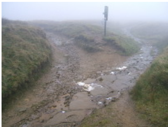
Water flowing off BW 92 onto Chapel Gate. No running water was seen on the Chapel Gate track continuing to the left of the fork. October 2016
