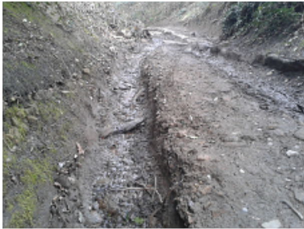
Damage to the surface: April 2016
