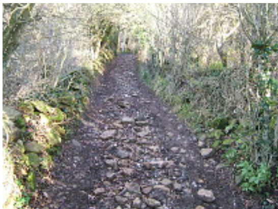
Poor surface which is unsuitable for horses: December 2015
