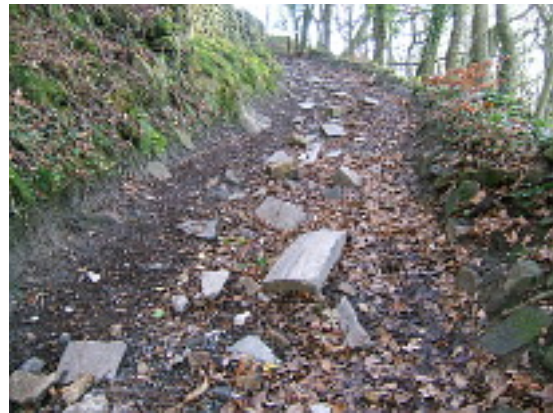
Poor surface: December 2015
