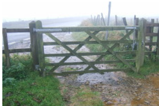
Water running off Chapel Gate onto the Sheffield Road. October 2016
