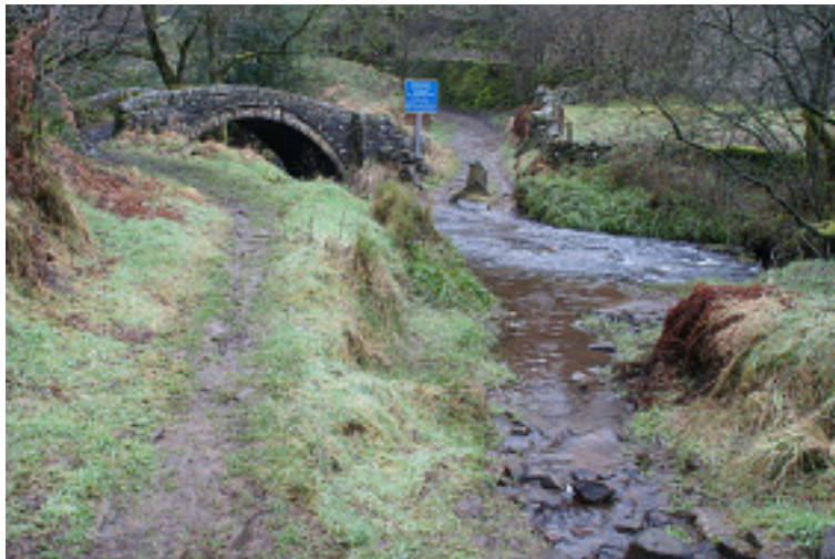
The packhorse bridge. The official path is on the left. The upright stone on the far bank was placed to stop vehicles using the ford.
