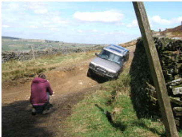
A deeply eroded section of Ramsden Road near Holmfirth. April 2016
