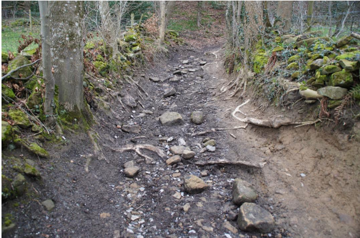
Jacob's Ladder in April 2018 with exposed tree routes, limited width and poor visibility at a bend
