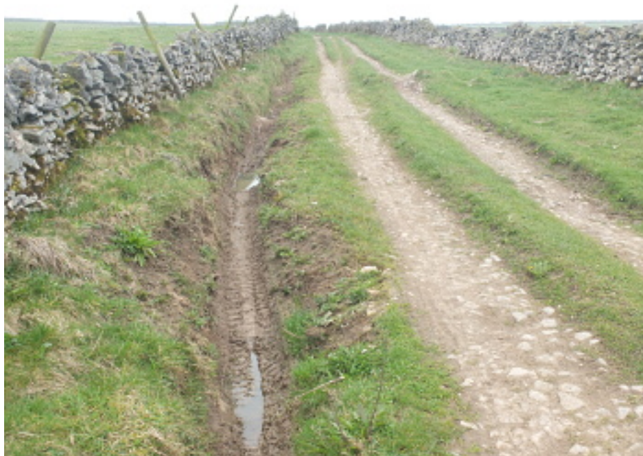
Tyre tracks clearly visible in a deep rut beside Sough Lane. Although not illegal as the actual BOAT is defined as being between the walls, such driving is unnecessary and unsightly. April 2019
