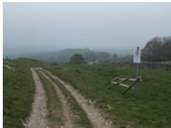
The top of the previous short cut. Although the barrier is damaged there were no visible signs of deviations from the track here.
