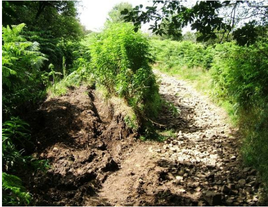
Off piste driving creating a parallel track August 2012
