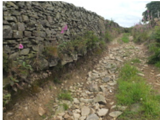
Foundations of walls being undermined. Photograph July 2015
