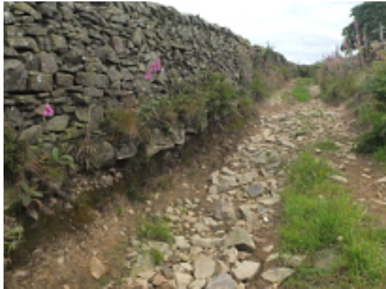
Limer Rake: Wall footings undermined. July 2015
