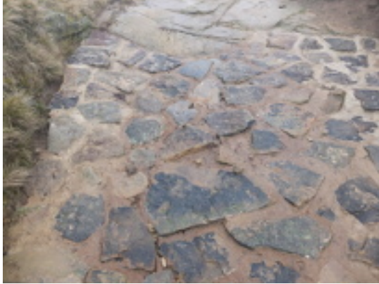
An obviously repaired section. January 2020
